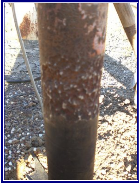
Before; Severe External Corrosion
