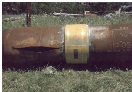
Note the bulging of the pipe outside the repair area.
